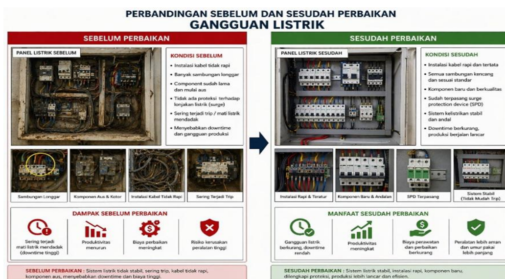
Figure 7. Electrical faults before repairs
